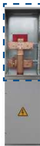
Busbars Compartment Scompato Sbarre Omnibus
